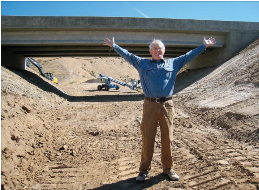
Ed Bottum celebrates the completion of a wildlife underpass on State Highway 21 near Boise. IDFG photos by Vicky Osborn
